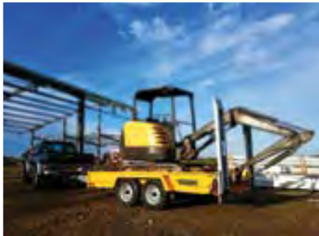
7h00 Delivery of a mini-excavator at the construction site of an industrial building.
